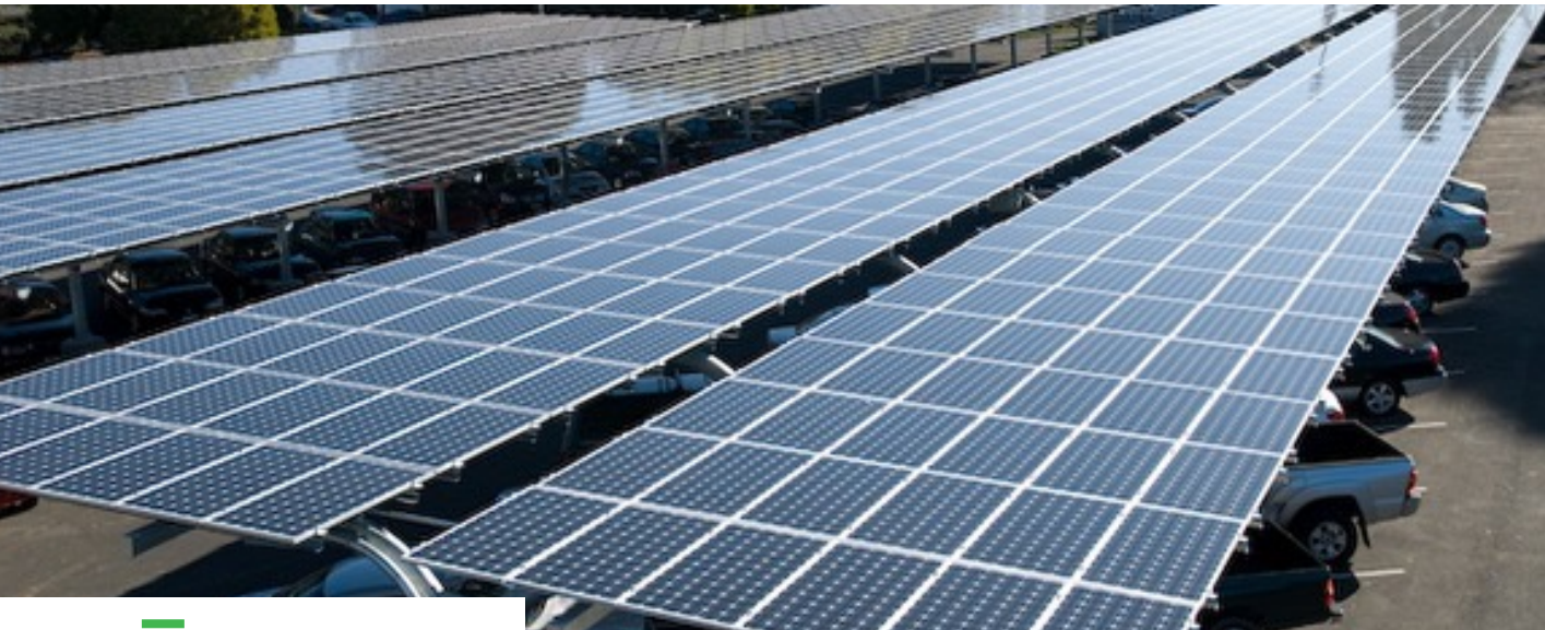
Solar panel parking
